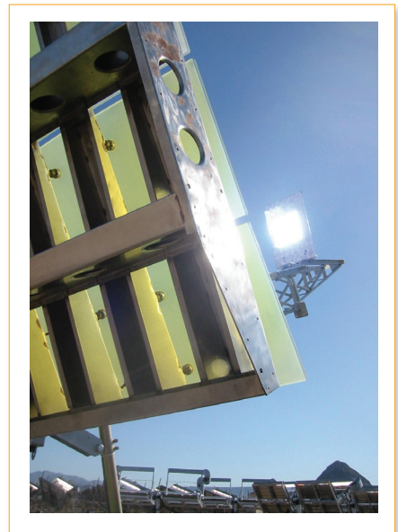
Figure 6 —Reflective facets, collector structure, and focused beam in target area.
