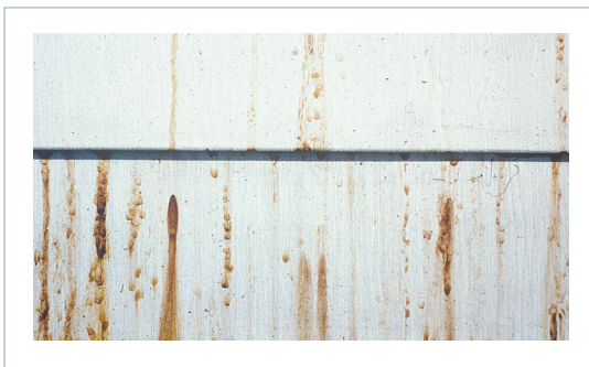
Figure 2 —Run-down extractive bleed.
