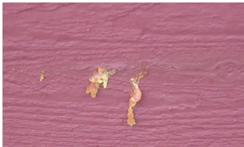
Figure 10—Localized pitch bleed.
