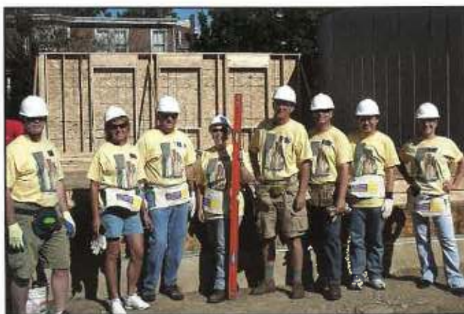
In Philadelphia, Rohm and Haas recently sponsored its second Habitat for Humanity House, with many employees contributing their own time to do the physical work.
